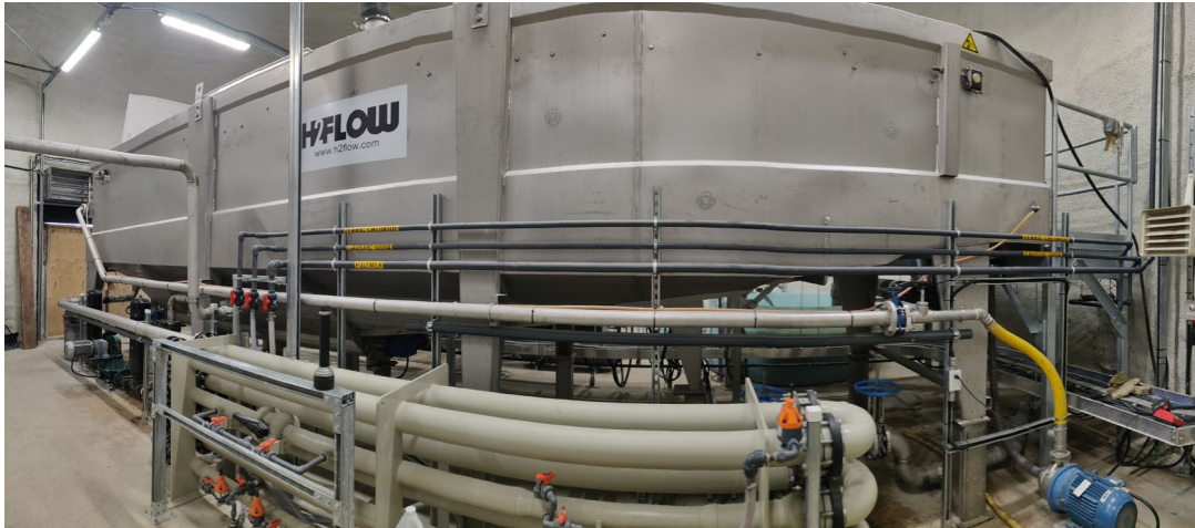
H2Flow DAF Unit and Pipe Flocculator
