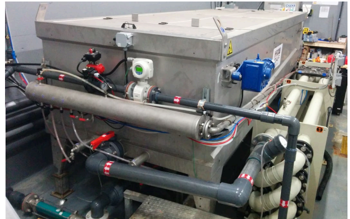
ALPHA 30 DAF and Flocculator
