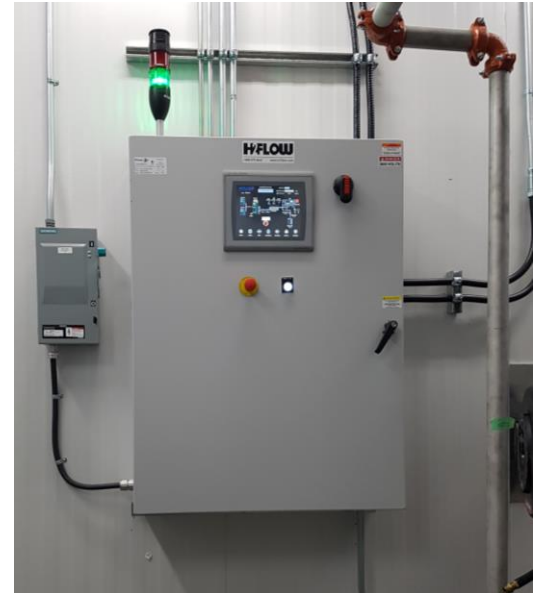
H2Flow PLC with HMI display
